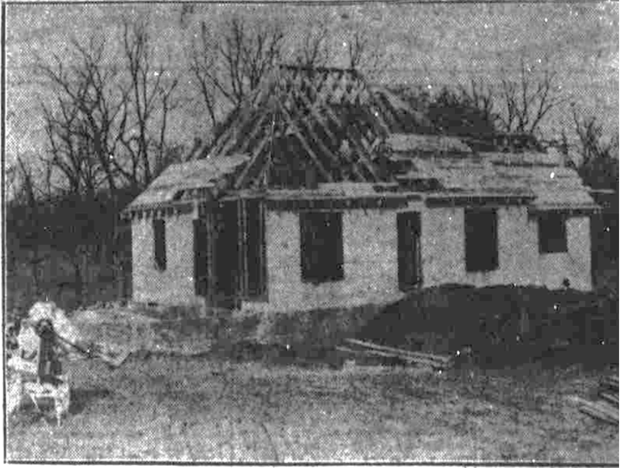
The Model Home going up in wood frame, before any masonry, The Nashville Tennessean , early 1927 (photographs by C. J. Burnell, January 30 and February 6, 1927). (Public domain.)
